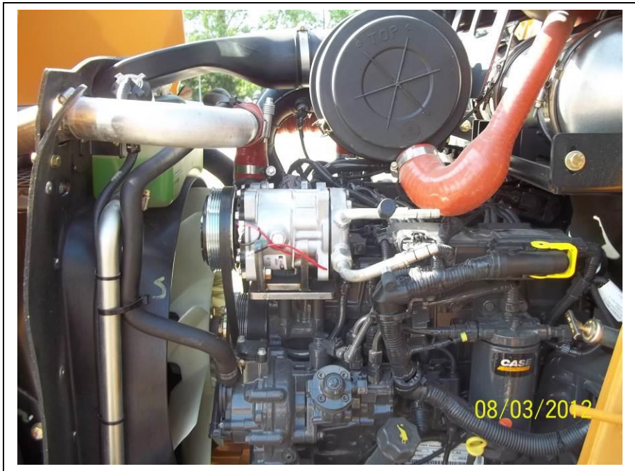
Compressor mount installed showing hose configuration
