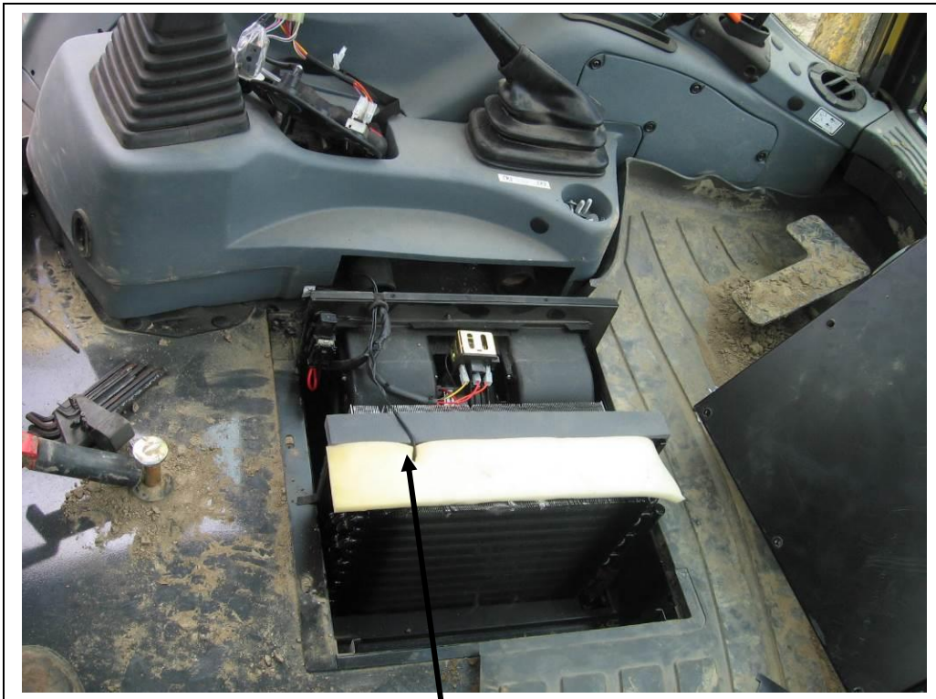
Thermostat probe inserted in the evaporator.
